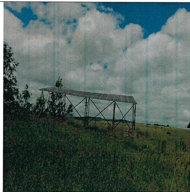
Solar Power water pumping system in Narok
